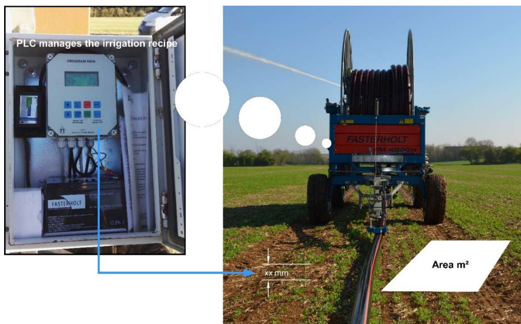
Figure 6: Existing installed technology to manage an irrigation recipe
