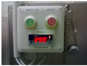
Photo 8: Equipment installed in the mixtures area.
