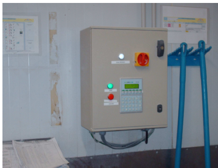
Photo 4: Electrical box installed in the mixtures zone with operator interface.
